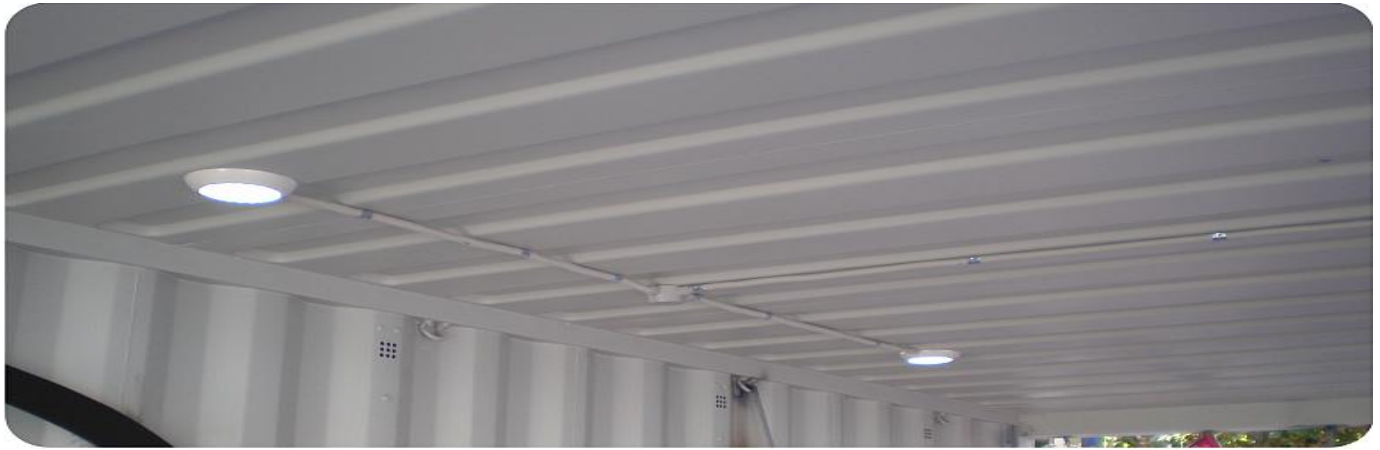
Container with two 200 lumen lights, Optional flexible conduit and junction box was included to run cable along roof
